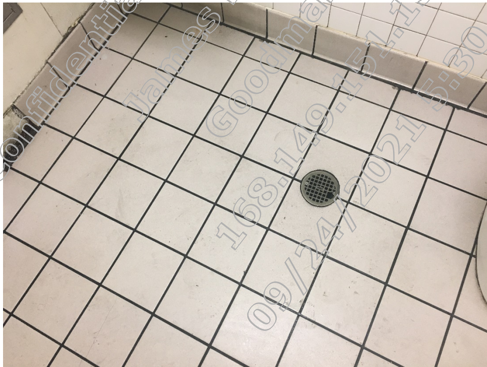
A total of six floor drains were located on the subject property: four at the car wash and two in the bathrooms of the convenience store.
