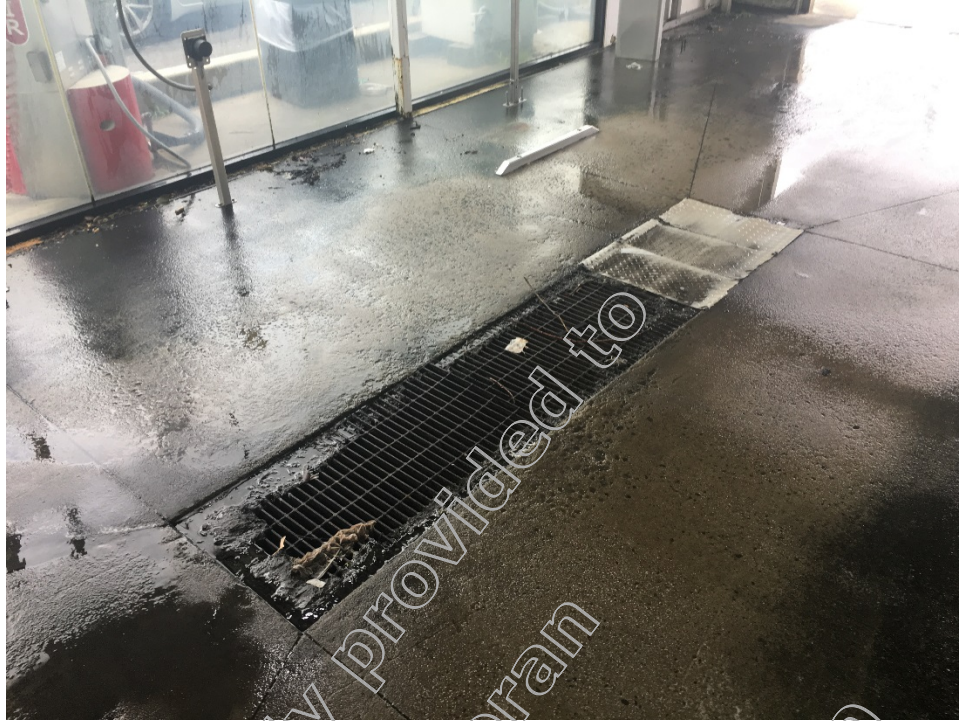
A total of six floor drains were located on the subject property: four at the car wash and two in the bathrooms of the convenience store.
