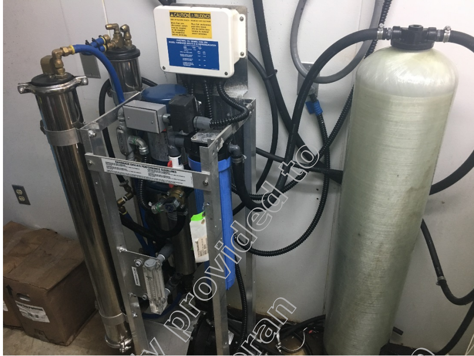
A 100-gallon tank of water with a filtration system for the car wash was observed.
