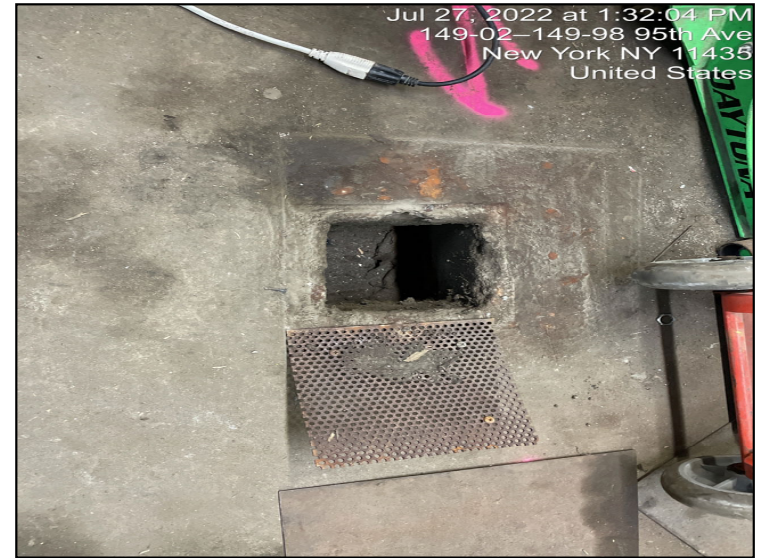
Photograph 6: Open floor drain prior in Lot 10 prior to collection of sample RI-SB-DRAIN.
