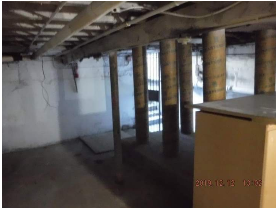
Photograph 3: View of Sump1 in the basement of 161-03 29 th Avenue (sump is under plywood cover at background). Support posts for former dry cleaning machine visible at right.
