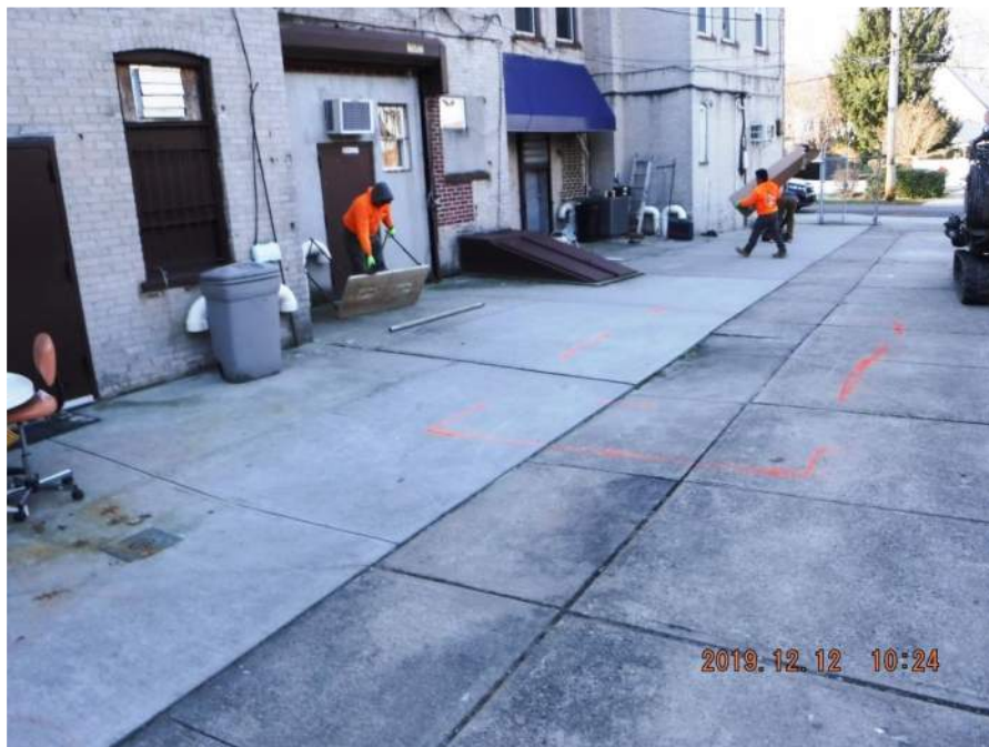
Photograph 2: Outline of the UST in red spray paint as established by the GPR survey. Photographer facing west.
