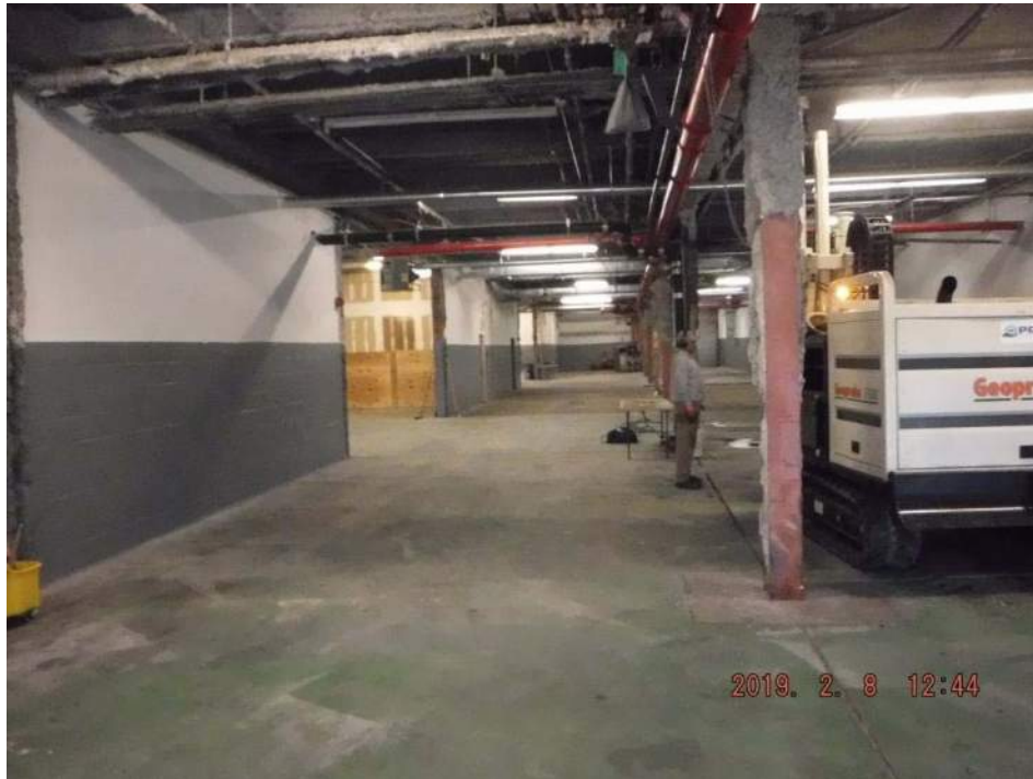
Photograph 7: Interior of the vacant ground floor of the two-story Site building. Installation of B9 shown.
