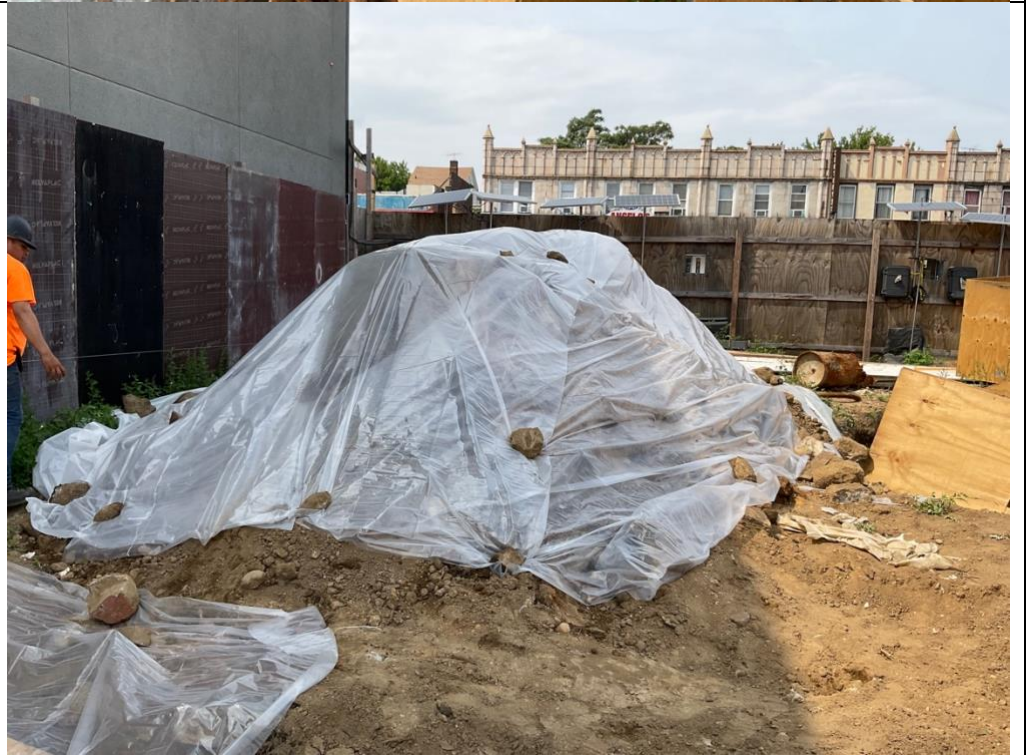
Photo 4 – The hazardous Stockpile in A1 at the end of the workday.
