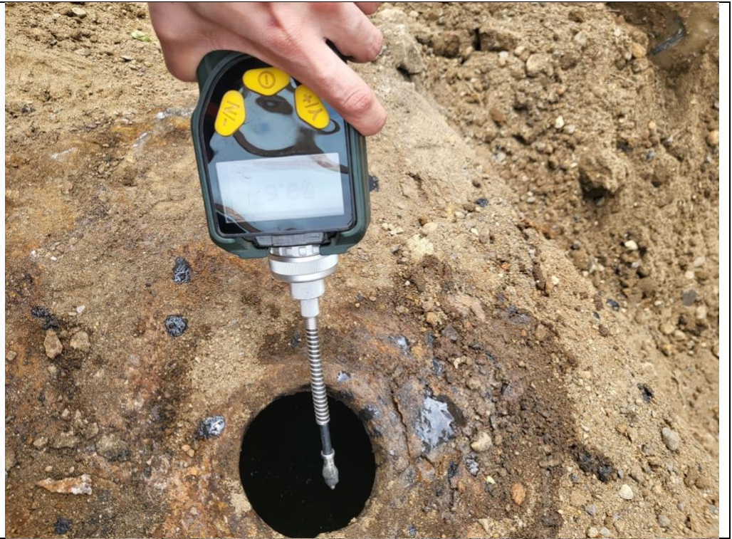
Photo 3 – PID reading inside of the tank. The tank is currently containing some waste oil without any spills.
