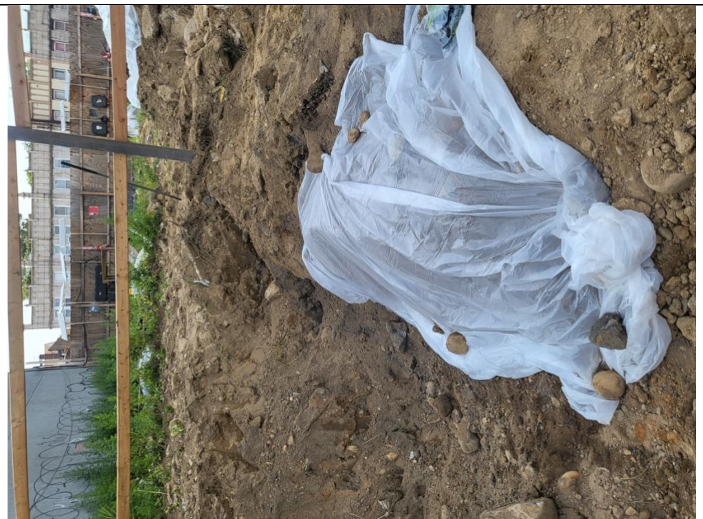
Photo 5 - Exposed UST have been covered by plastic tarp to prevent any potential contamination until its proper removal.
