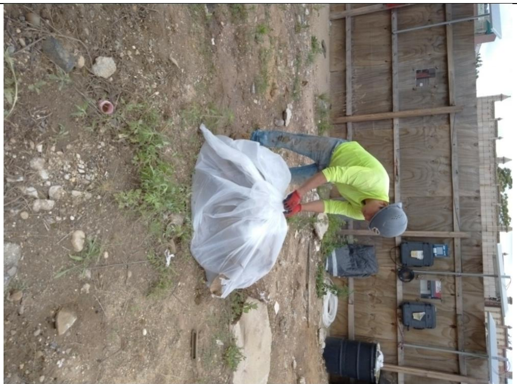
Photo 7 – The tank was moved and wrapped by a polyethylene sheet for a proper disposal.
