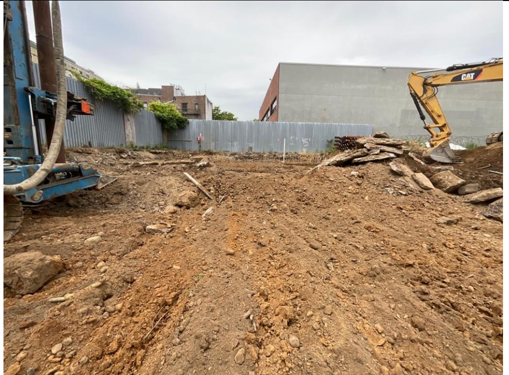
Photo 3 – Excavation area, 0-2 ft bgs, in the SW corner of the site, A3, A4, B3, and B4.
