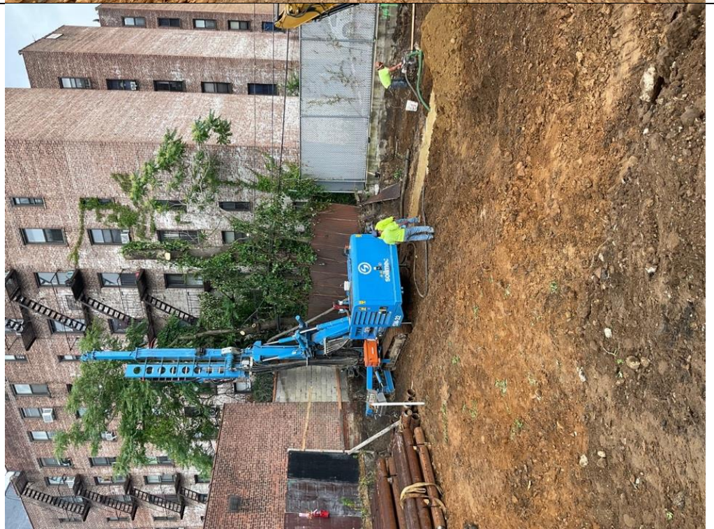
Photo 4 – Installing of 1 st shoring pile in the SE corner of the site.
