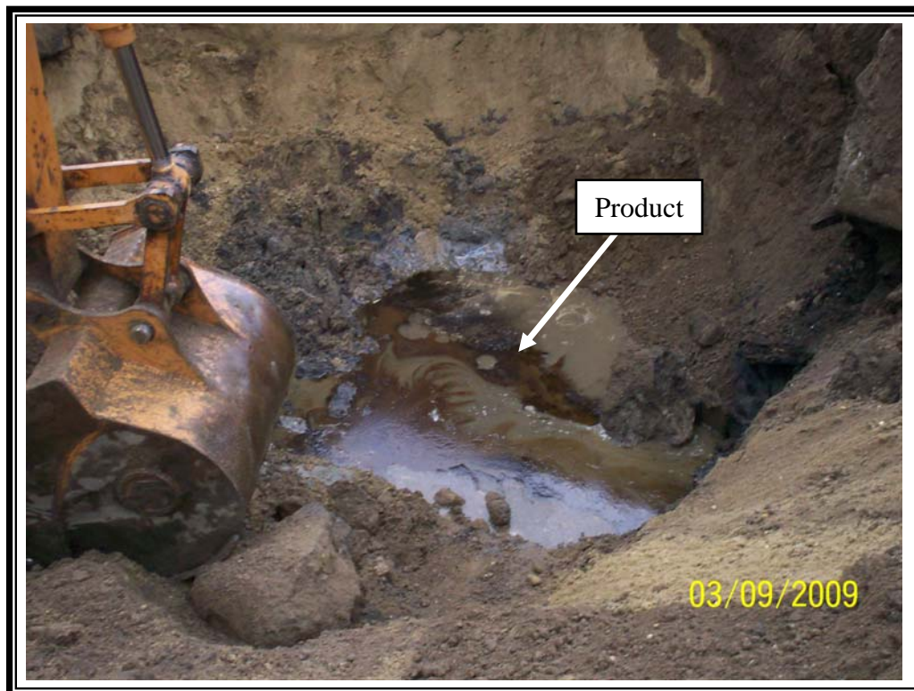
Photo 2: View of test pit TP-3 (southwestern corner of Site, near MW-4s/MW-4i well cluster), showing free-phase petroleum product encountered.
