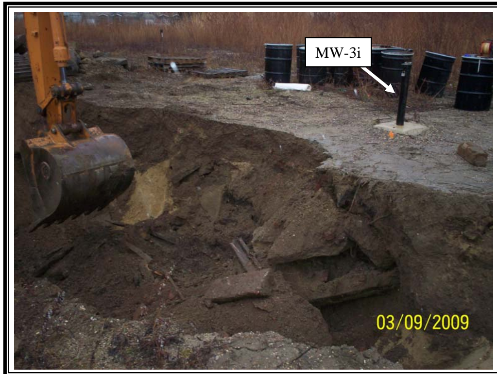
Photo 1: View of south wall of test pit TP-3 (southwestern corner of Site, near MW-4s/MW-4i well cluster), showing buried concrete blocks, metal, and other debris.
