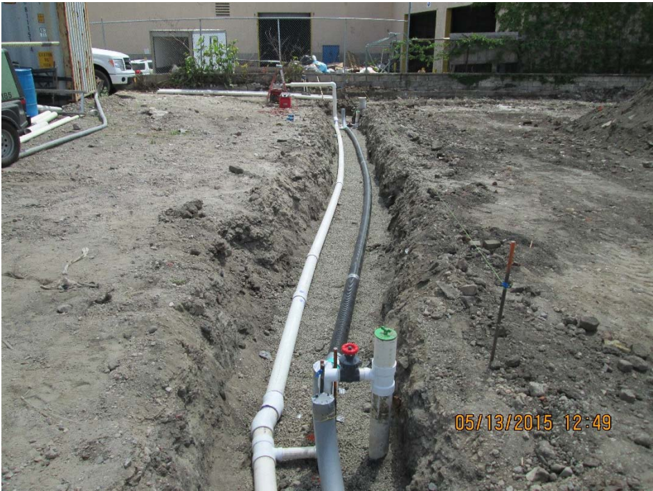
Photograph 2: VER piping in TF-3 trench on RAD II
