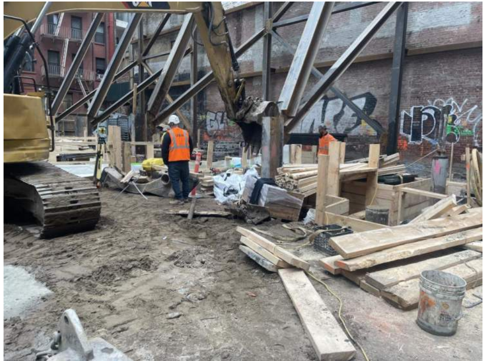
Photo 2: View of Urban backfilling along timber lagging in WC04 with previously imported pipe sand (facing southeast).
