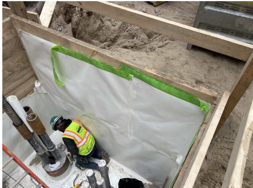
Photo 2: Urban installing waterproofing around pile caps in the southern part of the site (facing southeast).
