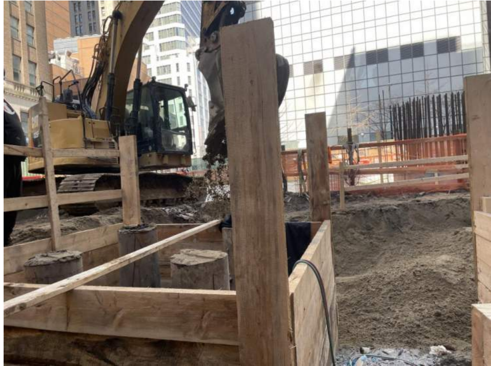
Photo 1: Urban backfilling around timber lagging with previously imported clean pipe sand (facing northeast).
