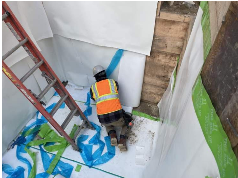
Photo 2: Urban installing waterproofing in the southern portion of the site (facing southwest).
