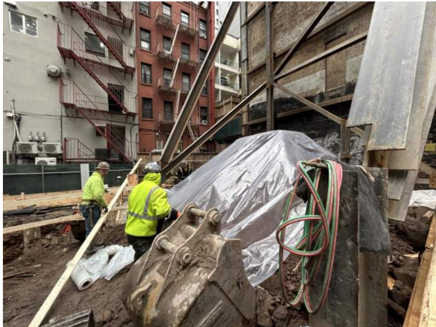
Photo 4: Urban covering the soil/fill stockpile in grid WC05 with polyethylene sheeting at end of workday (facing southeast).
