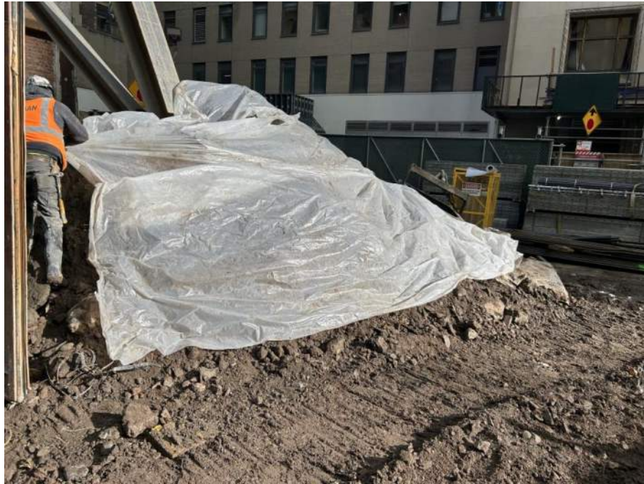
Photo 3: View of Urban covering the stockpile in WC04 with polyethylene sheeting at the end of the workday (facing west).
