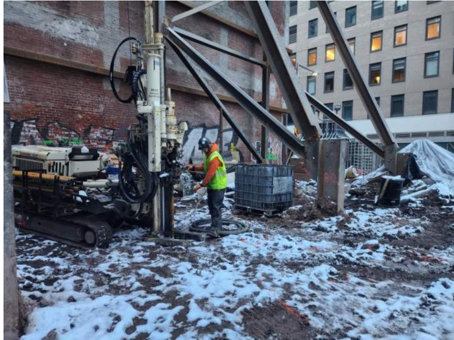
Photo 1: View of Brookside and Coastal injecting batch-mixed PetroFix® in the southern part of the site (facing southwest).
