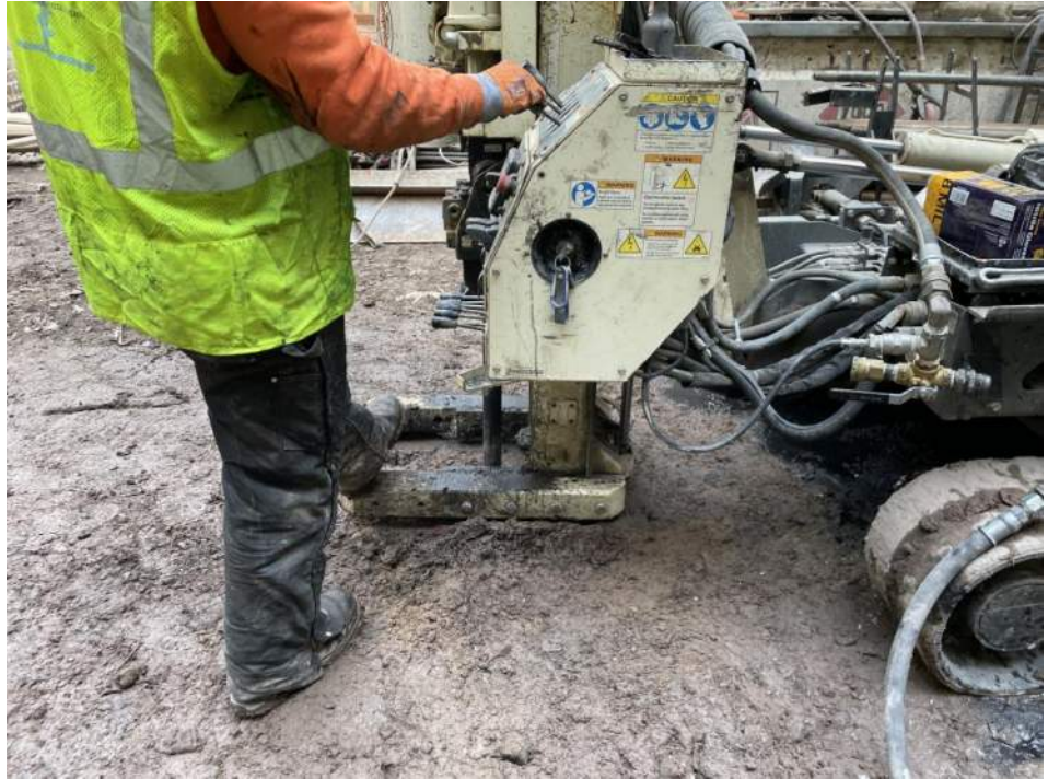
Photo 1: View of Brookside and Coastal installing an injection point in the southern part of the site (facing east).
