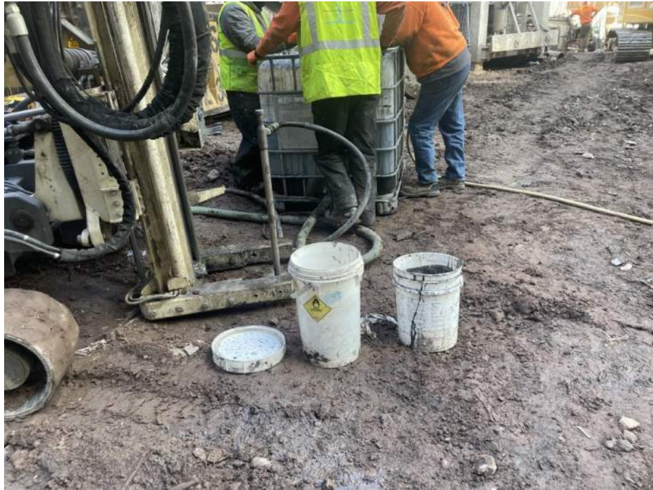
Photo 3: View of Brookside and Coastal installing an injection point in the southern part of the site (facing northwest).
