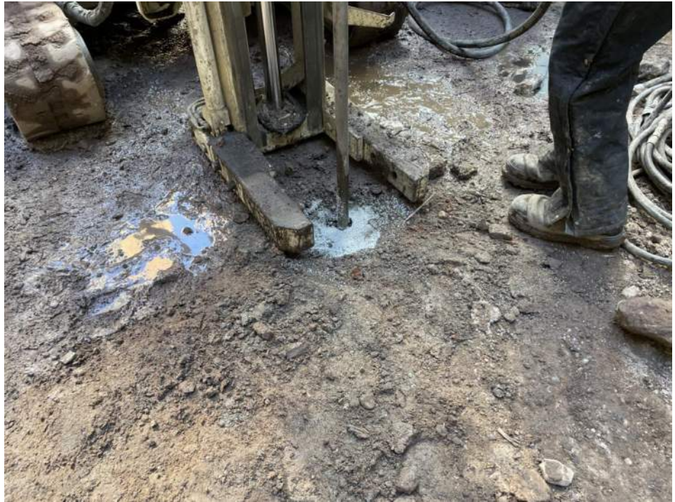
Photo 3: Overhead view of an injection point with surface bentonite seal installed by Brookside and Coastal.
