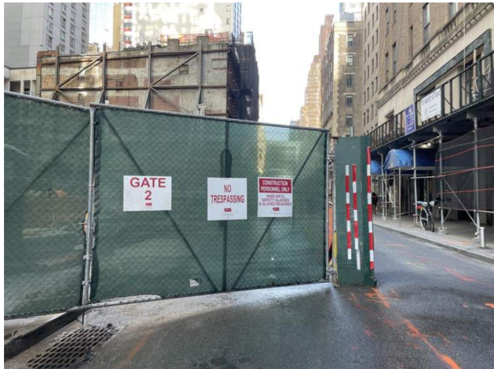
Photo 4: View of the site entrance/exit at the corner of Washington and Carlisle Streets at the end of the work day (facing south).
