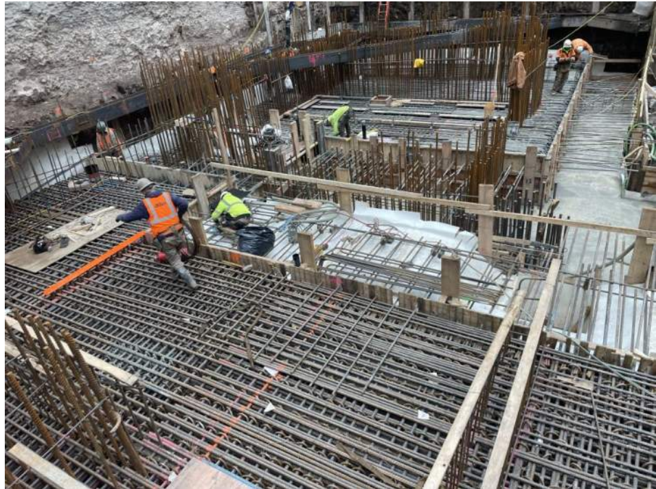
Photo 2: Urban installing waterproofing/vapor barrier in the central part of the site facing southeast).
