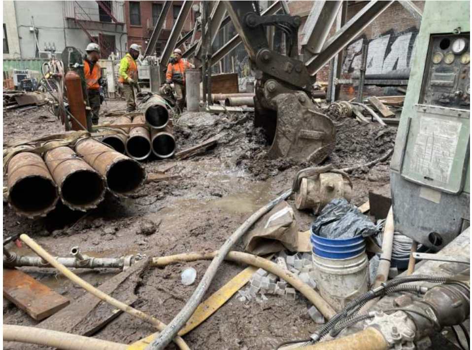
Photo 1: Urban excavating soil/fill in the central part of grid WC04 (facing southeast).
