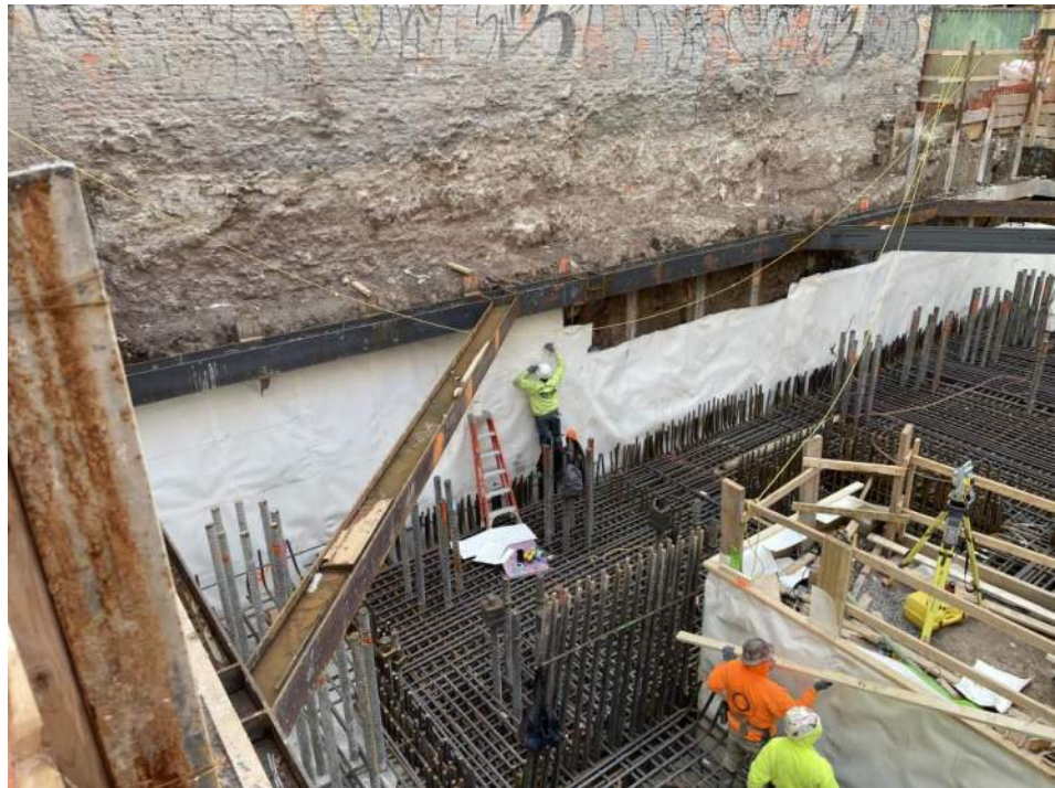
Photo 2: Urban installing the waterproofing/vapor barrier membrane in the eastern part of the site (facing southeast).
