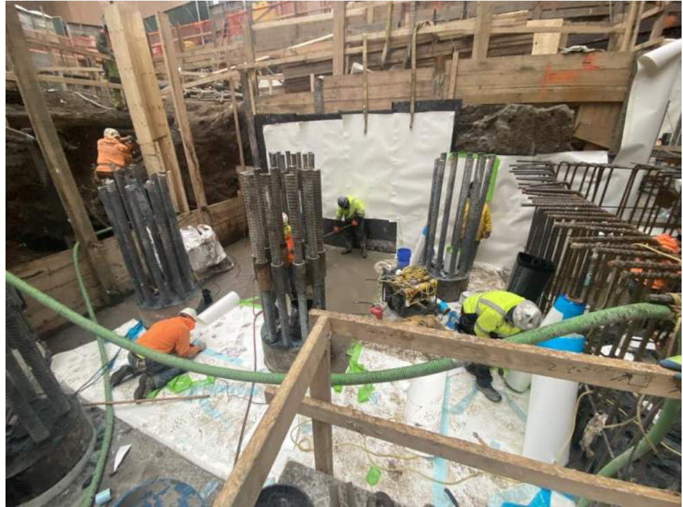
Photo 1: Urban installing waterproofing/vapor barrier membrane in the central part of the site (facing north).
