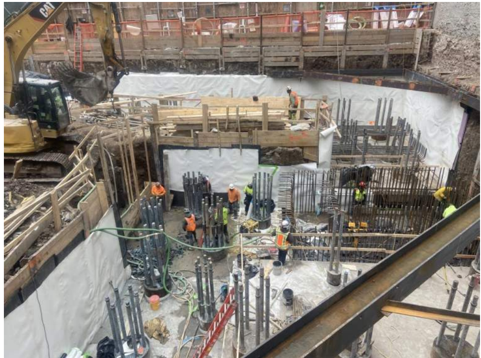
Photo 2: Urban using a jackhammer to remove concrete in the central part of the site (facing north).
