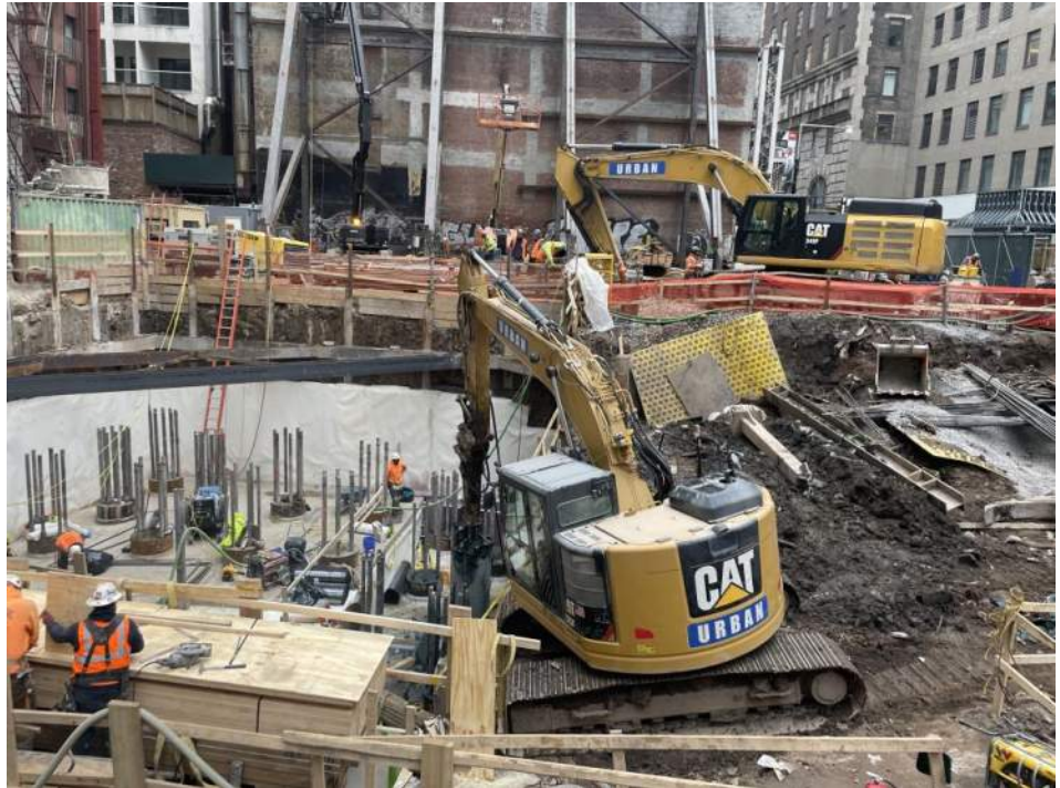
Photo 2: Urban removing concrete in the central part of the site (facing south).
