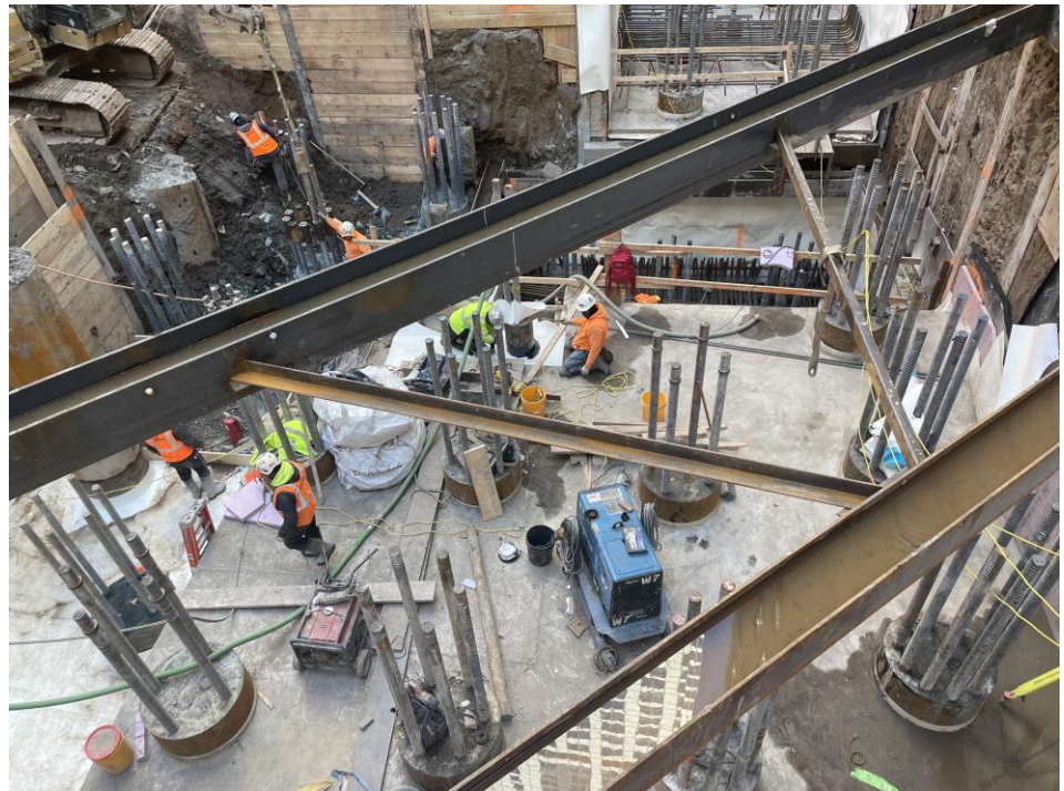
Photo 2: Urban installing waterproofing/vapor barrier membranes in the central part of the site (facing north).
