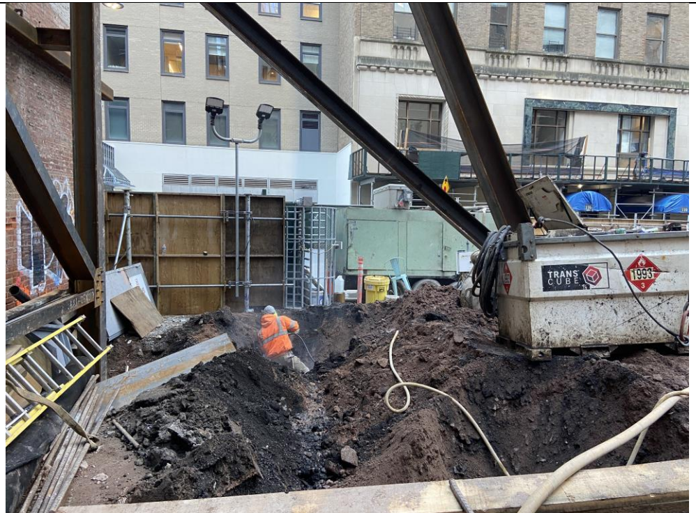
Photo 2: Urban jackhammering the former foundation in the southwest part of WC04 to prepare for the installation of caisson casing.
