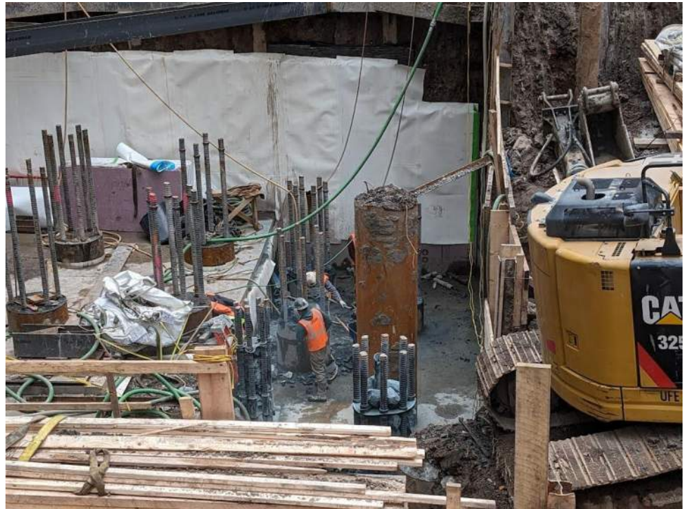
Photo 2: View of Urban using a jackhammer to remove concrete from existing caissons in the central-southern side of the excavation area (facing east).
