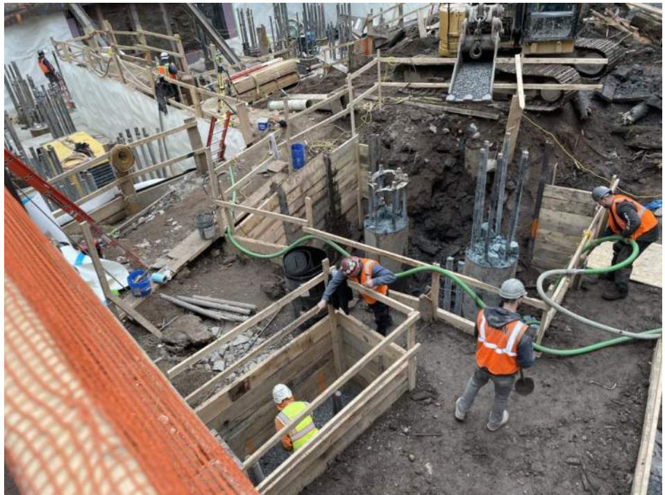
Photo 2: View of Urban backfilling previously imported 0.75-inch stone in grid WC02_20-25 (facing southeast).
