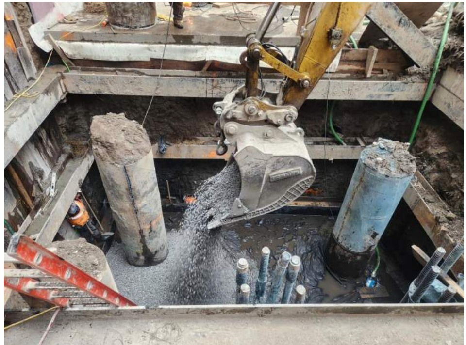
Photo 2: View of Urban backfilling previously imported 0.75-inch stone in grid WC06_30-35 (facing south).
