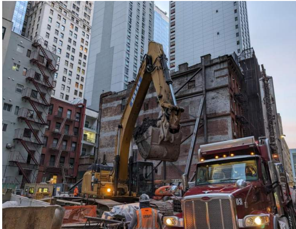
Photo 2: View of Urban loading a truck with soil/fill for off-site disposal (facing southeast).
