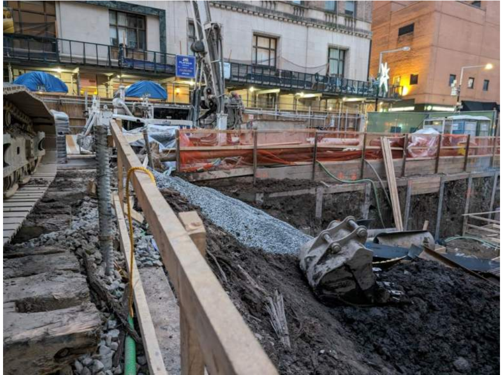
Photo 1: View of imported 0.75-inch stone stockpiled in the southwestern part of grid WC02 (facing west).
