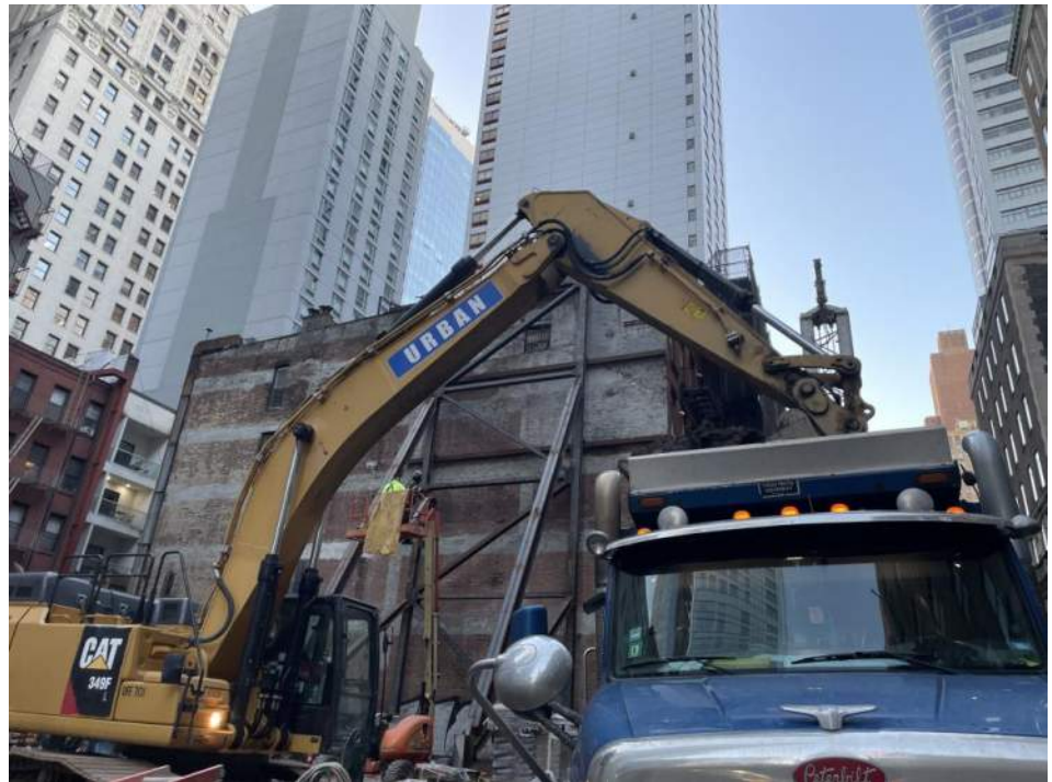
Photo 2: View of Urban loading a truck with soil/fill for off-site disposal (facing southeast).
