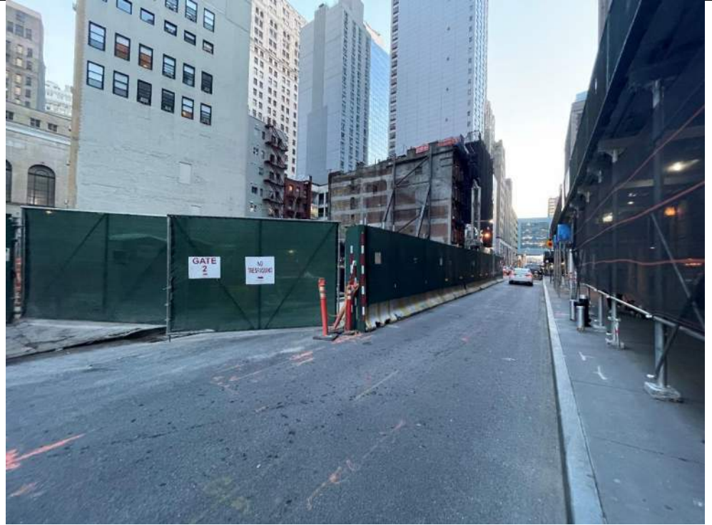
Photo 3: View of the site entrance/exit on the corner of Carlisle Street and Washington Street at the end of the workday (facing south).
