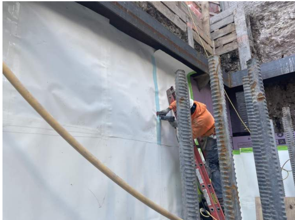
Photo 2: View Urban applying waterproofing in the northeastern part of the site (facing northeast).
