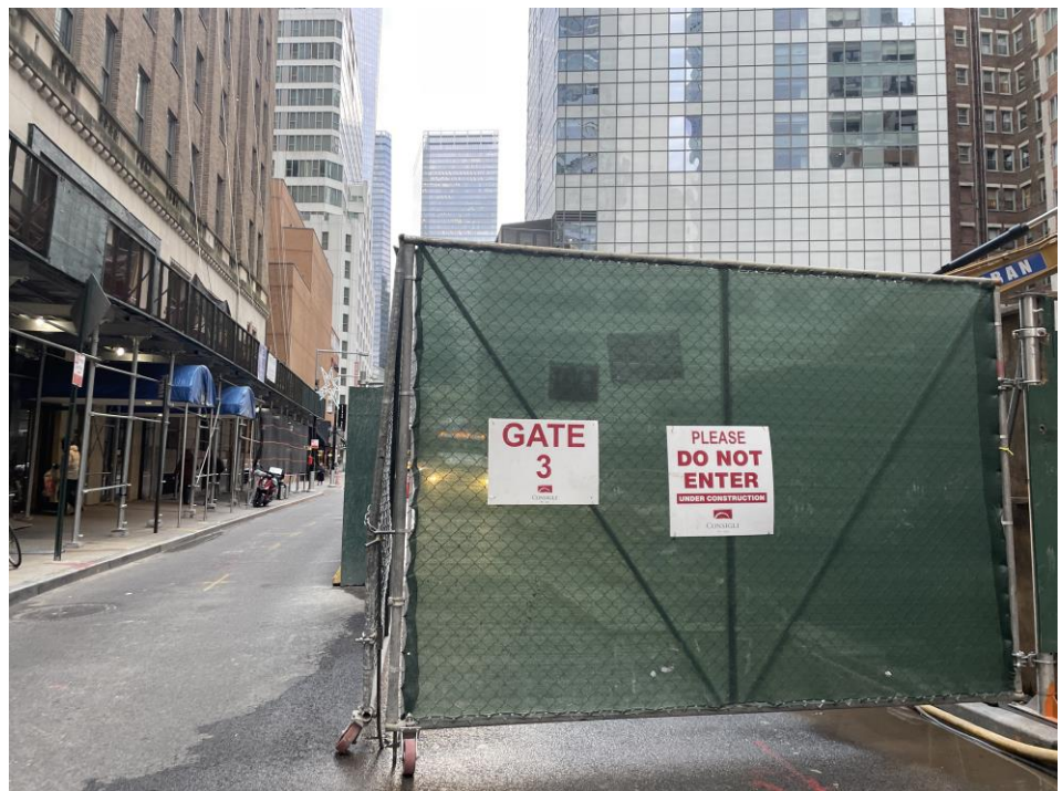
Photo 4: View of the site entrance/exit on Washington Street at the end of the workday (facing north).
