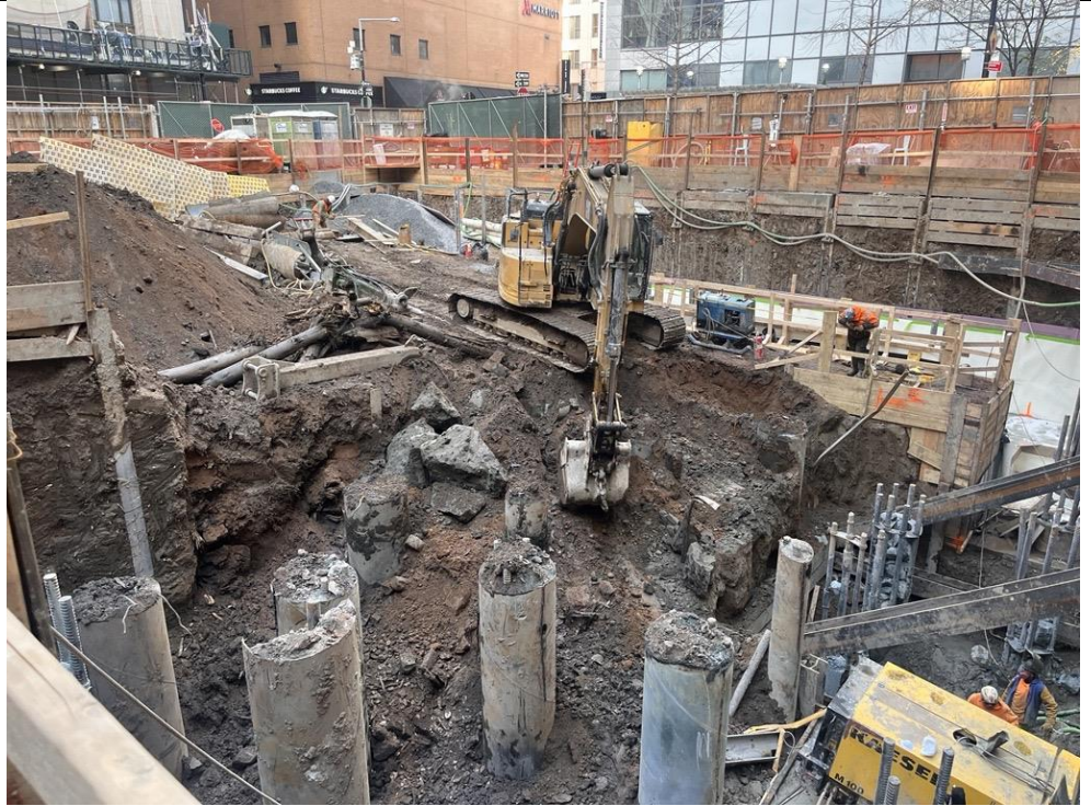
Photo 1: View of Urban excavating soil/fill in the central part of the site (facing northwest).
