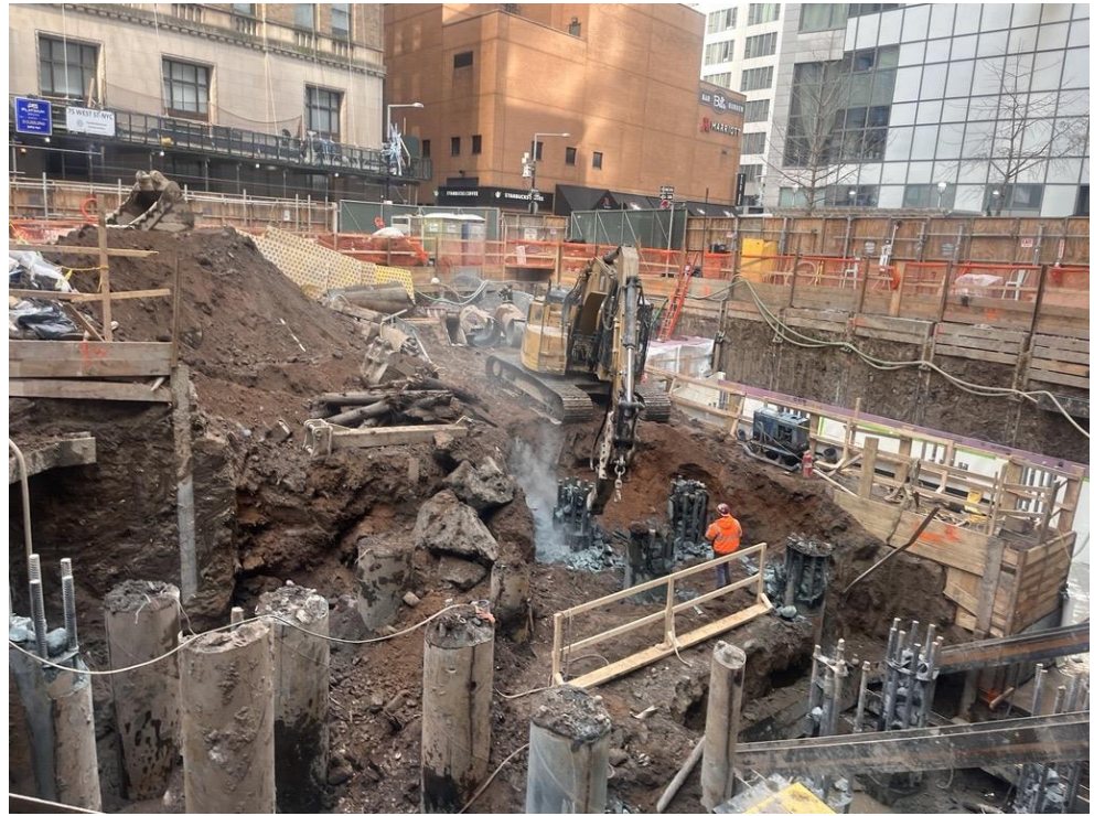
Photo 3: View Urban removing concrete from existing caissons in the central part of the site (facing northwest).
