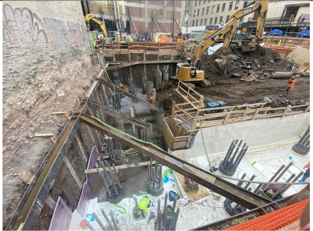
Photo 1: View of Urban installing waterproofing/vapor barrier membranes in the northeastern part of the site (facing south).
