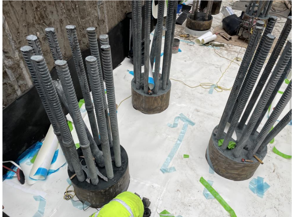
Photo 1: View of Urban installing waterproofing/vapor barrier membranes in the northeastern part of the site (facing southwest ).
