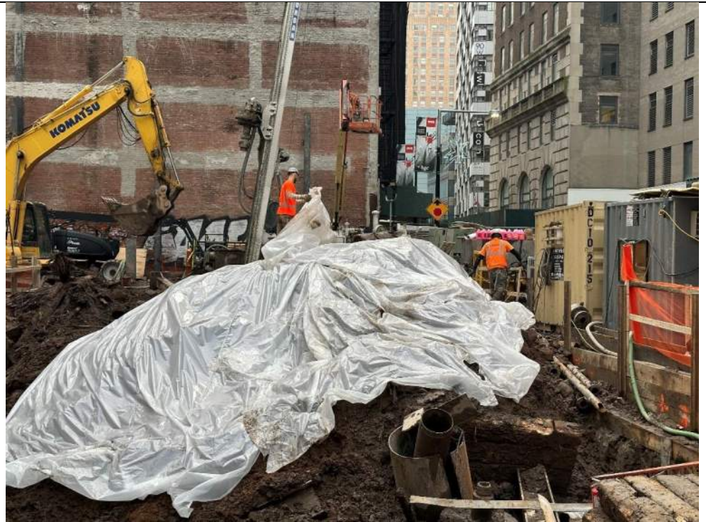
Photo 3: View of Urban covering soil/fill stockpile in grid WC02 with polyethylene sheeting (facing south).
