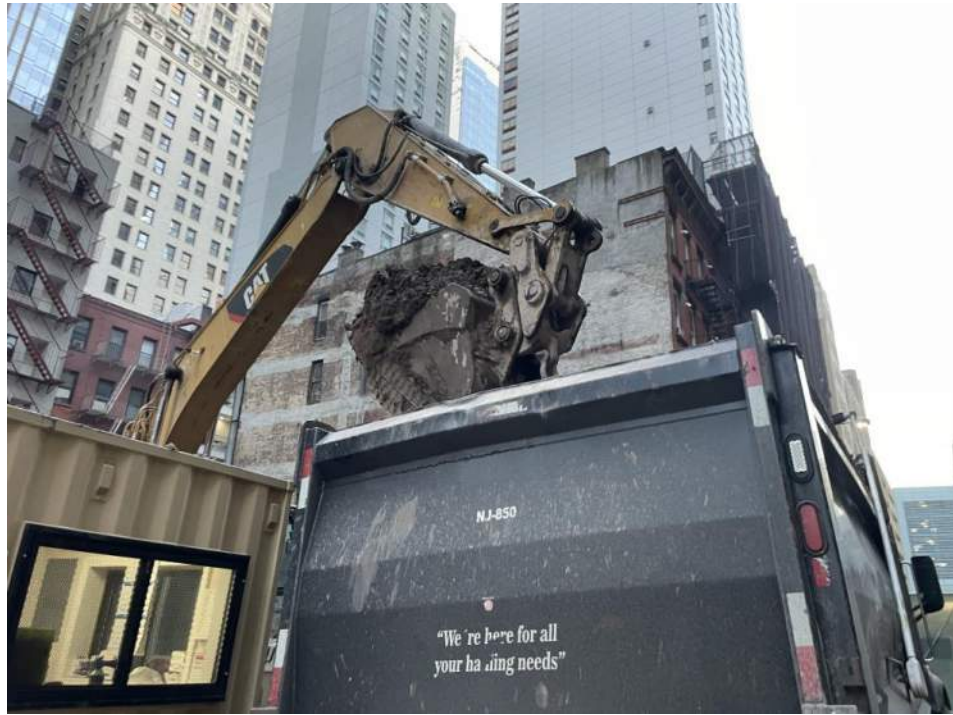
Photo 1: View of Urban loading a truck with soil/fill for off-site disposal (facing southeast).
