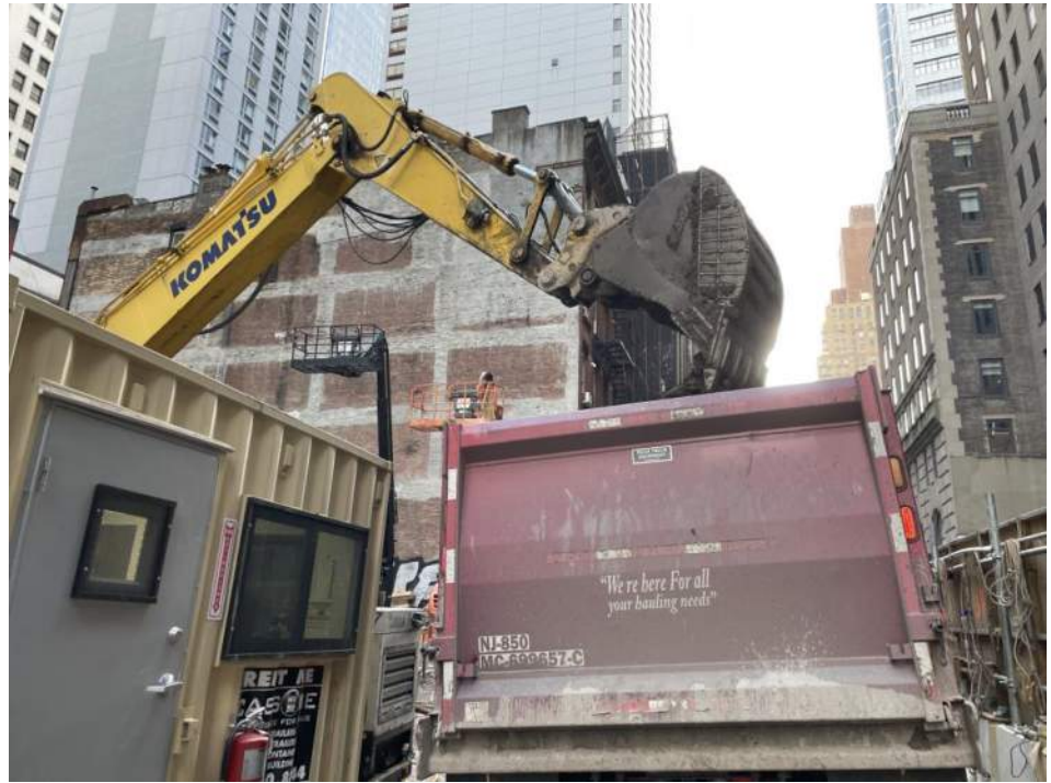
Photo 1: View of Urban loading a truck with soil/fill for off-site disposal (facing south).
