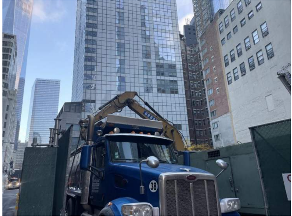
Photo 1: View of Urban loading a truck with soil/fill for off-site disposal (facing northeast).
