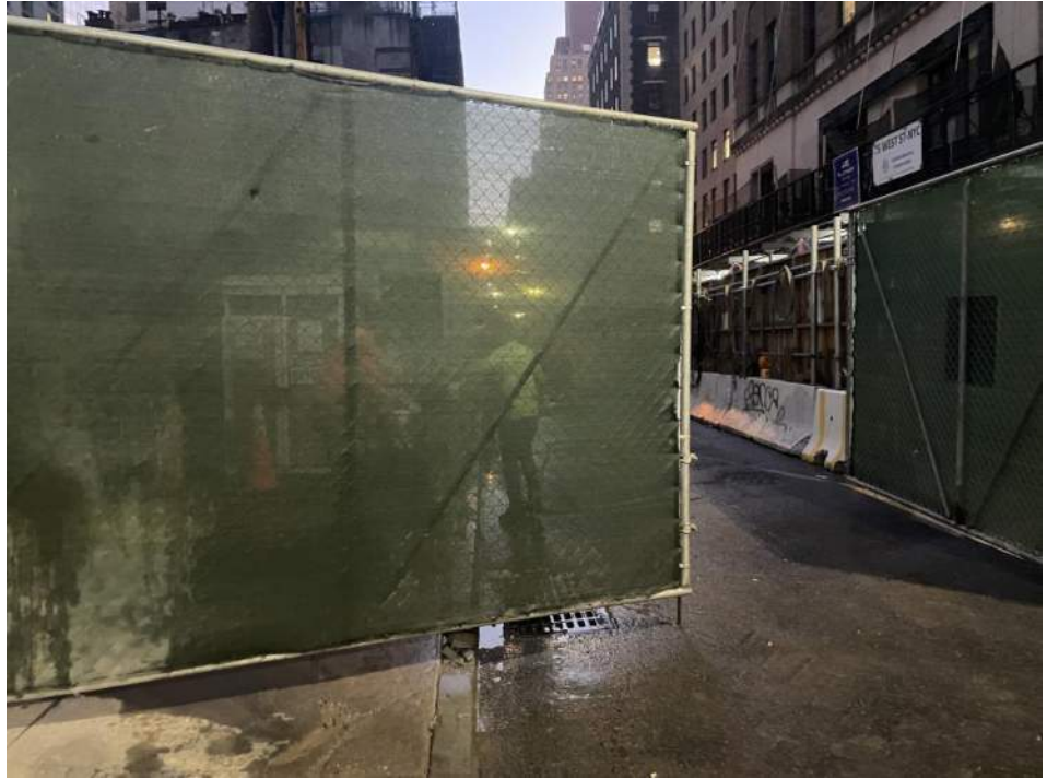
Photo 3: View of the site entrance/exit at the corner of Carlisle and Washington Street at the end of the work day (facing southeast).
