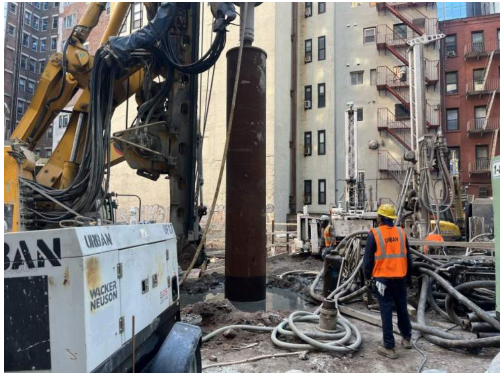
Photo 2: View of Urban installing a casing for a caisson in the western part of the site (facing east).
