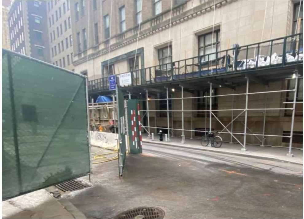
Photo 3: View of the site entrance/exit at the corner of Carlisle and Washington Street at the end of the work day (facing southwest).
