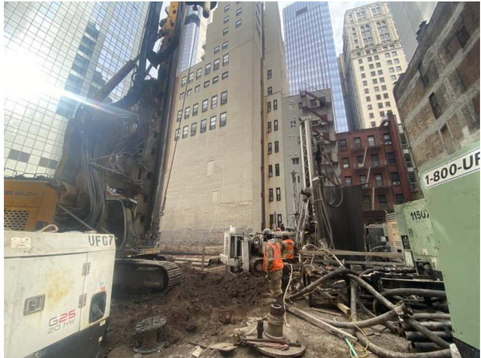
Photo 1: View of Urban preparing to drill in the northwestern part of grid WC04 (facing east).
