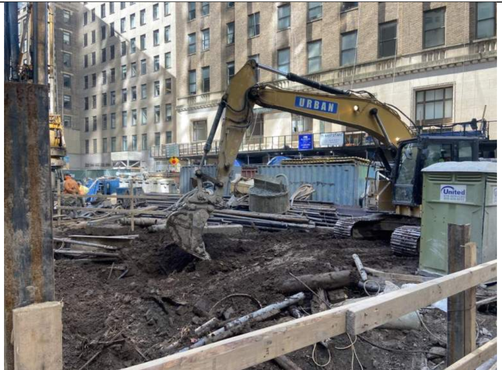
Photo 2: View of Urban excavating soil in grid WC02 in the western part of the site (facing southwest).
