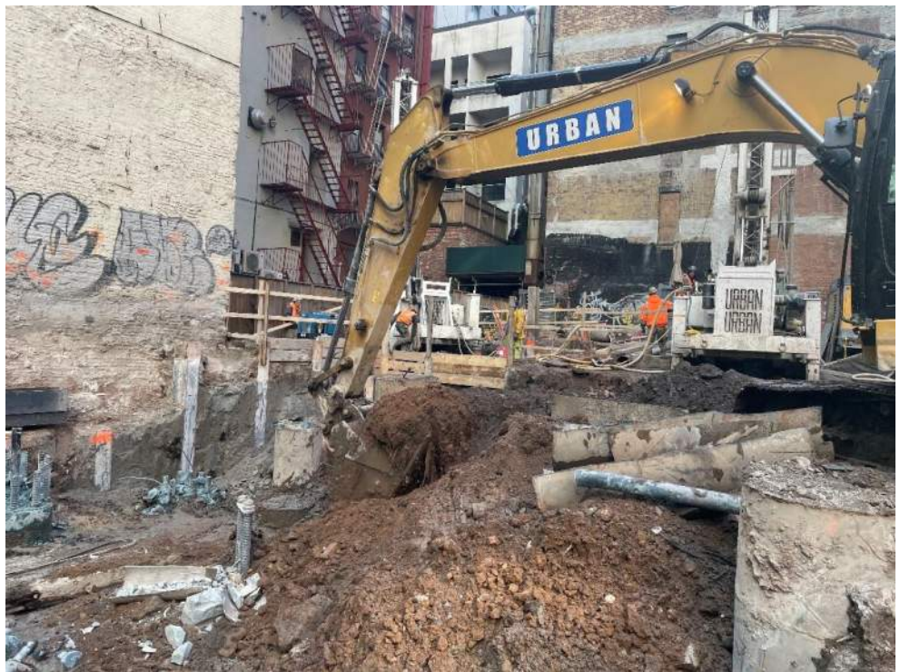
Photo 2: View of Urban excavating soil in grid WC03 in the eastern part of the site (facing southeast).
