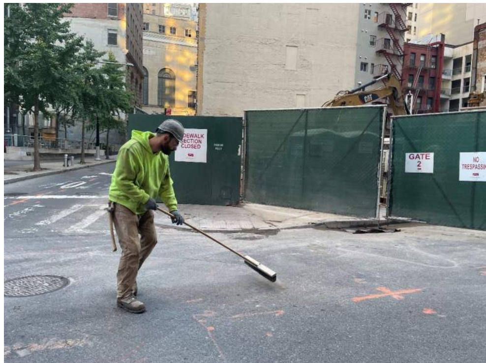
Photo 4: View of Urban sweeping the site entrance/exit at the corner of Carlisle and Washington Street at the end of the work day (facing east).
