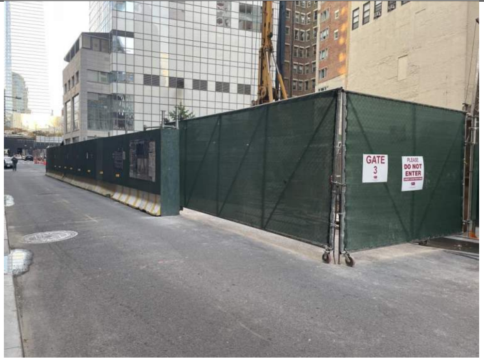
Photo 3: View of the site entrance/exit along Washington Street at the end of the work day (facing northeast).
