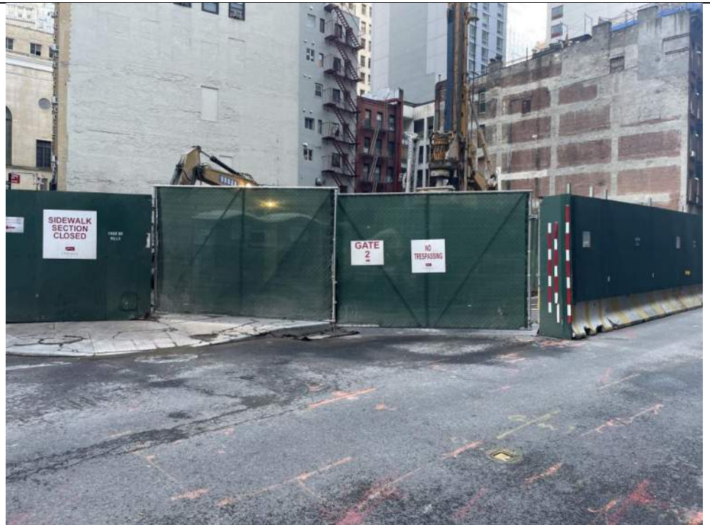
Photo 4: View of the site entrance/exit at the corner of Carlisle and Washington Street at the end of the work day (facing southeast).
