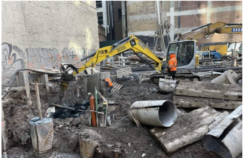
Photo 2: View of Urban breaking up concrete while using a hose for dust suppression (facing southeast).
