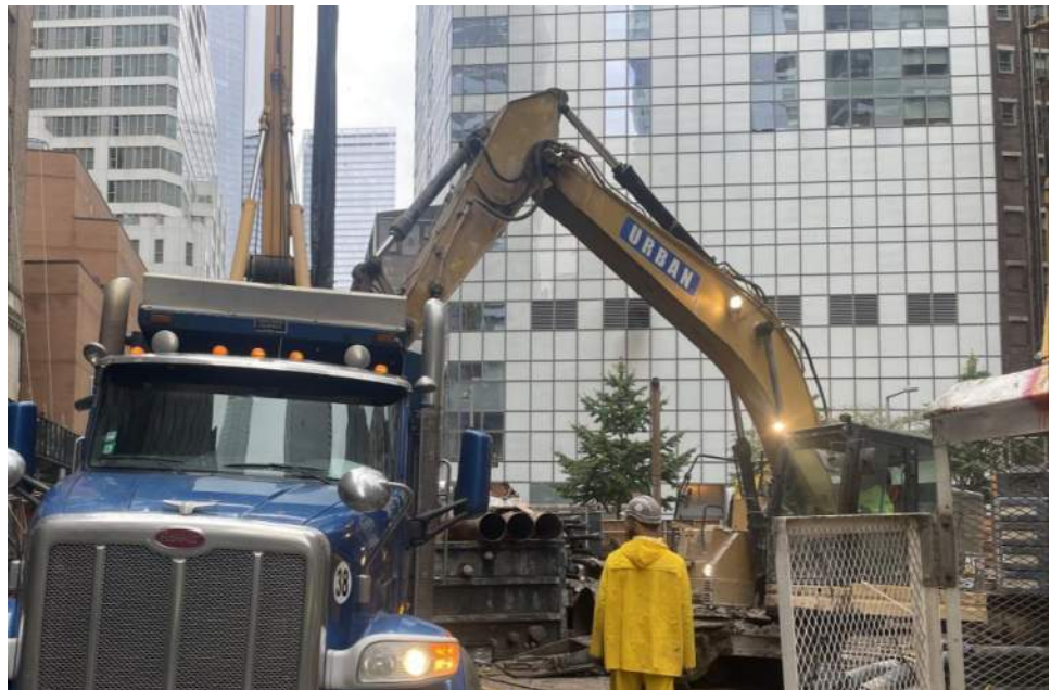
Photo 2: View of Urban loading truck with soil/fill for off-site disposal (facing north).
