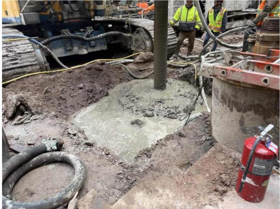
Photo 1: Urban installing soil-mix columns as part of the ISS in the southern part of the waste characterization grid WC04 (facing northeast).
